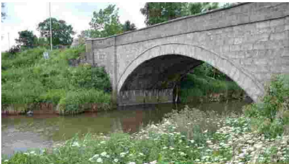
The bridge over the Urie requires a cycleway /pedestrian bridge.
